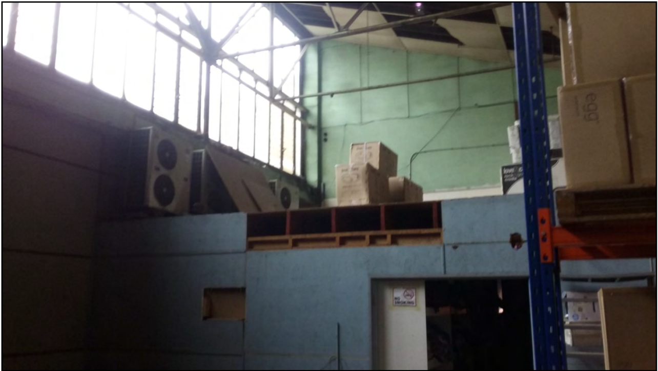
Photograph 7 – Air conditioning unit within rear warehouse, as observed on 19.12.2017
